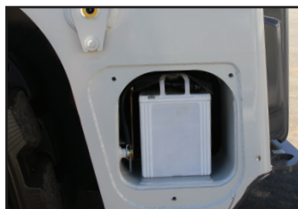
Battery Access Panel
